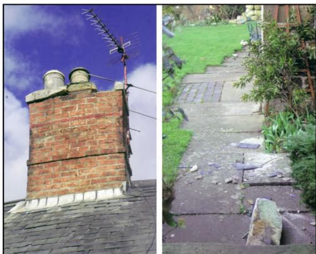
Figure 3. Earthquake damage to John Aram's house, where limestone coping fell from the chimney into the front garden.
